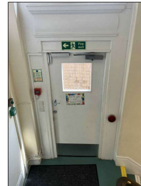
Internal door and frame to be replaced like for like by design.
