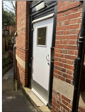
Existing door to be replaced. Design like for like with a material change from timber to steel.
